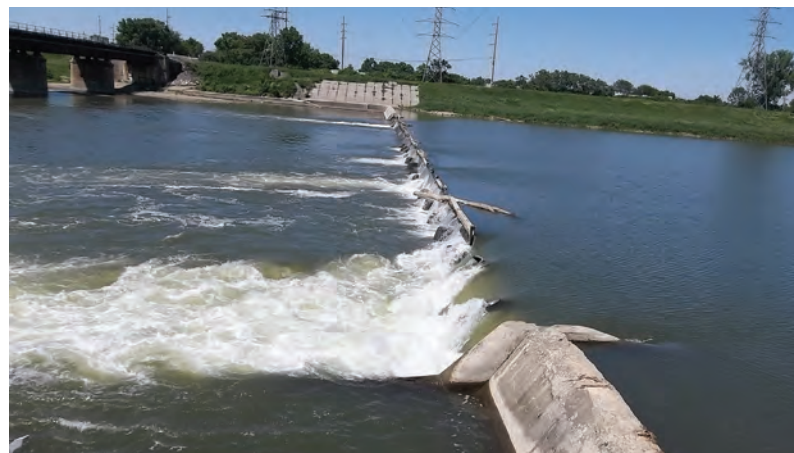
Tait Station low dam needs $5 to $8 million in repairs.
